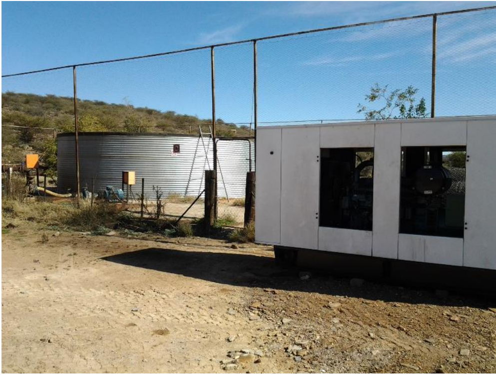
Figure 11: Raw water line pressure booster unit viewed towards the south west. The diesel power generator with no provided secondary containment is evident in the forefront.
