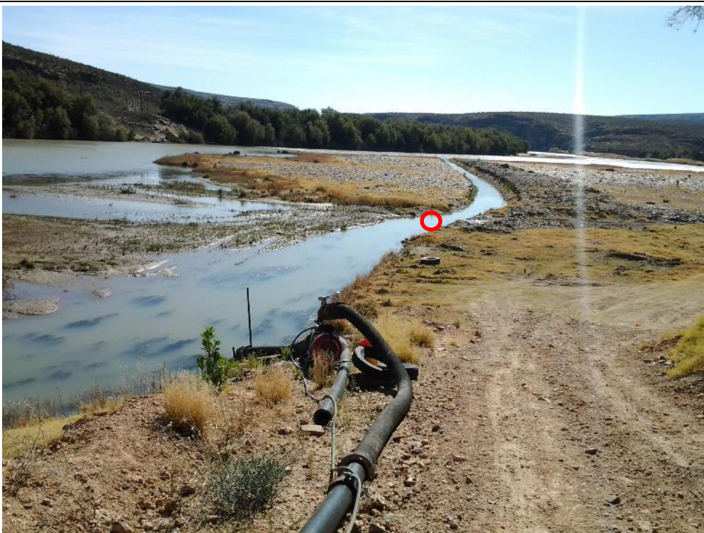
Figure 10: Raw water pump station on the banks of the Orange River viewed towards the north. Location of sample TSW01 downstream of the Thunderflex operation is indicated by the red circle.
