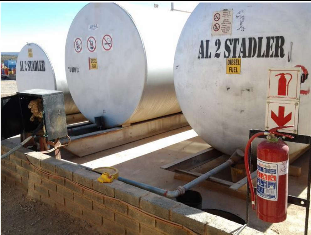
Figure 16: Diesel AST farm with the dispensing unit on the left.
