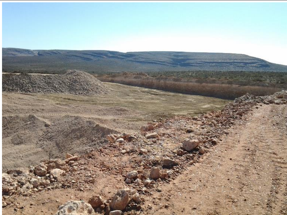
Figure 6: Prospecting trench with backfilling progressing from the left and trench void on the right.
