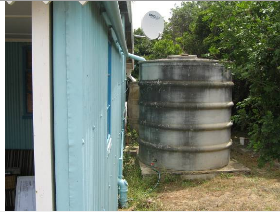
Photo 14: Two rainwater tanks and the conservancy tank on north-facing side of cottage
