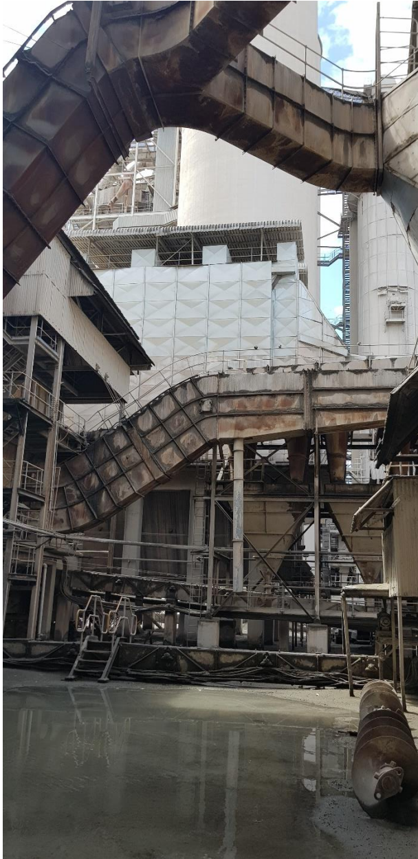
Figure 3: Example of Associated Infrastructure (Electrofilter)
