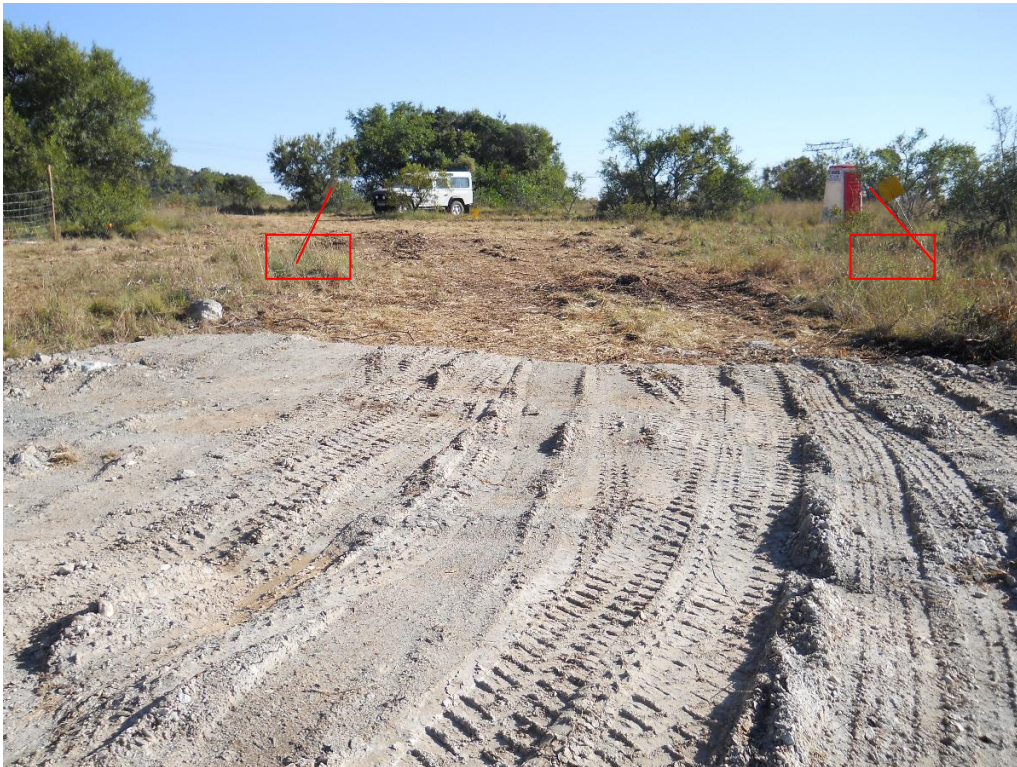
Fig 1. In the image above it is clear that the access road to the tower foundations just misses two of the graves, indicated in red.
