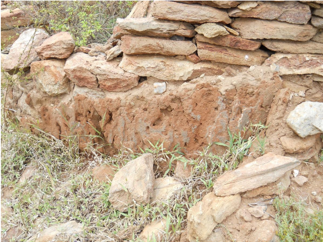
Fig 8. Some of the units still contain clay plastering on the external as well as internal surfaces. The approximate co-ordinates for this structure are 23°54'18.80"S 29°36'46.80"E.
