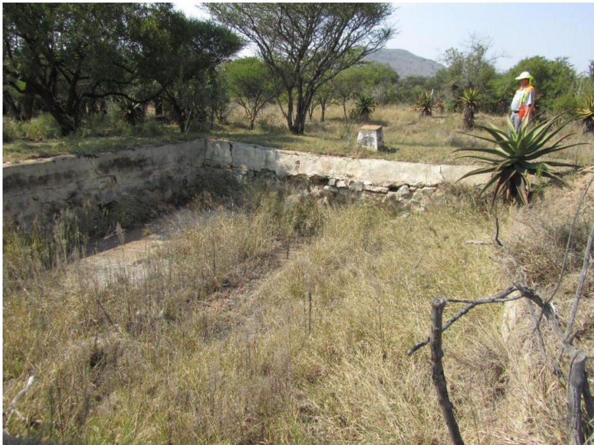
Figure 14. The sunken concrete reservoir.
