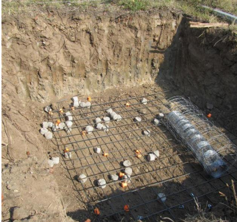
Figure 5. The second foundation of Tower 198. The soil colouring and texture differs markedly from the foundation (Fig 4) and is more clayey.
