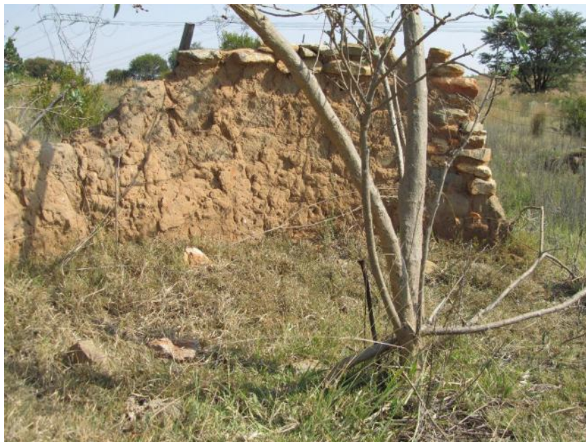
Figure 6. S24°00'23.8" E29°43'6". This homestead consists of a combination of square and circular stone walls. The square structures are built of clay bricks while the circular structures consist of stone and dagma walls plastered with clay. This was probably a farm labourer's homestead. The difference in building material could be due to later additions.
