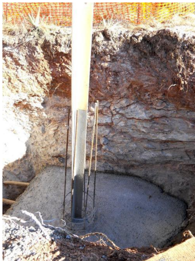
Figure 9. The commencement of the casting process. The archaeologist was on site during this process. No damage was done to the grave.
