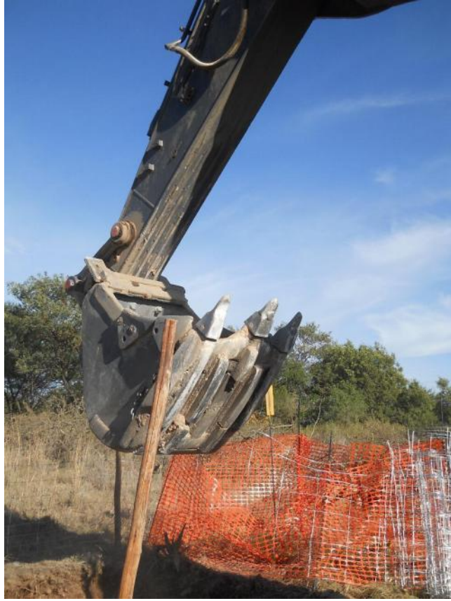
Figure 4. Great care was taken during excavation to prevent damage to the grave: when the bucket teeth blunted and made excavation not only difficult but also endangered the grave, another excavator replaced the previous, larger one.
