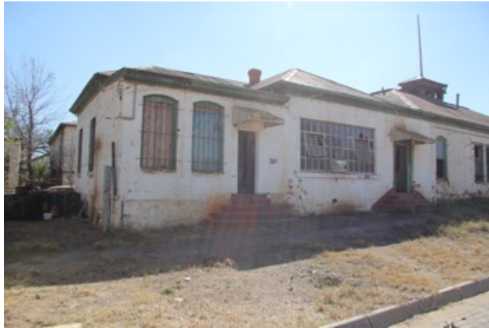
Figure 7: The original Office Building at Simmer and Jack. The building is disused and currently labelled as a hazard due to lack of maintenance.
