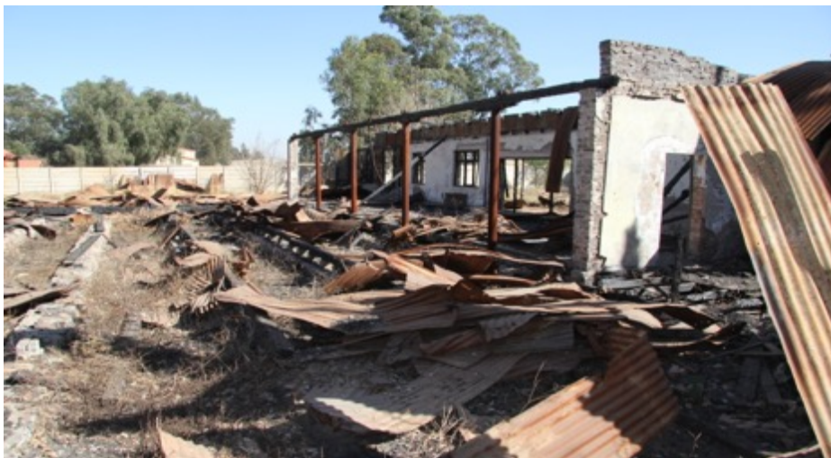
Figure 4: Remains of historical building at Simmer and Jack. The building was destroyed by fire.
