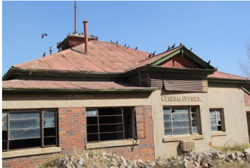
Figure 10: Section of the original Office Building at Simmer and Jack which is in poor and hazardous state earmarked for demolition.
