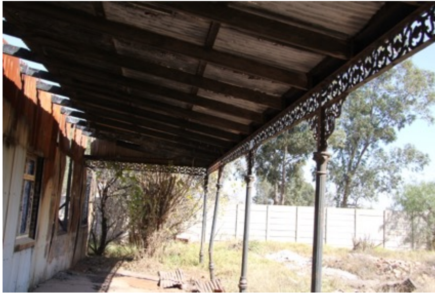
Figure 5: Remainder of verandah of historical building that was destroyed by fire.
