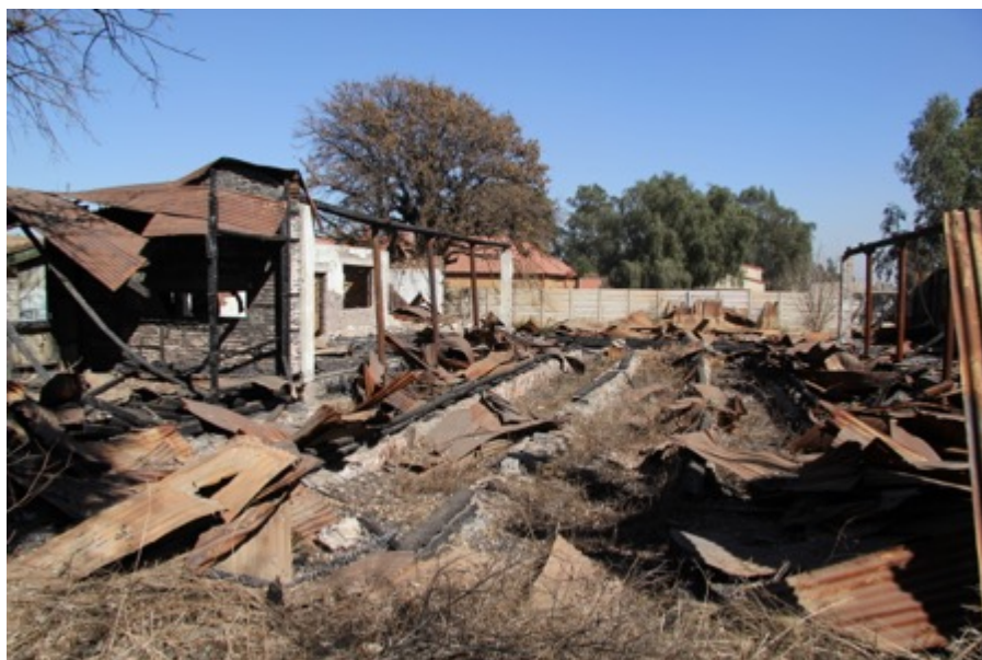
Figure 3: Remains of bunt-down building at Simmer and Jack site affected by proposed extension of the land fill (Source: Ekurhuleni).
