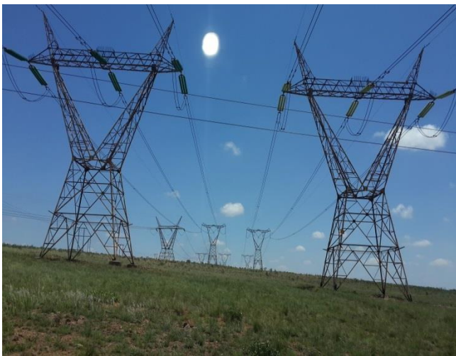
Photo # 3 : Eskom power lines through the site. On the northern Boundary
