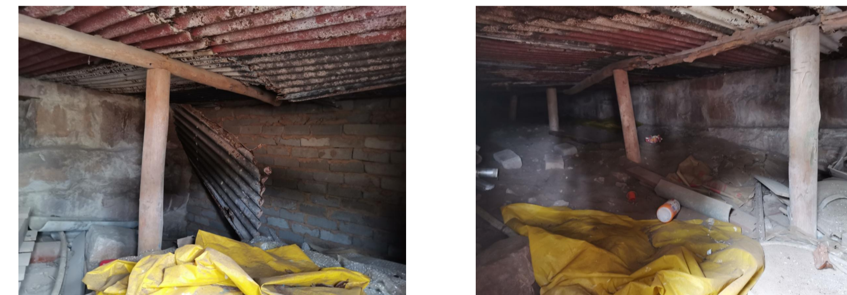
GENERAL CONDITION OF SUSPENDED SLAB UNDER VERNADAH - INDICATING PERMANANT CORRUGATED SHUTTERING AND GUMPOLE PROPS WITH WOOD BORER DAMAGE
