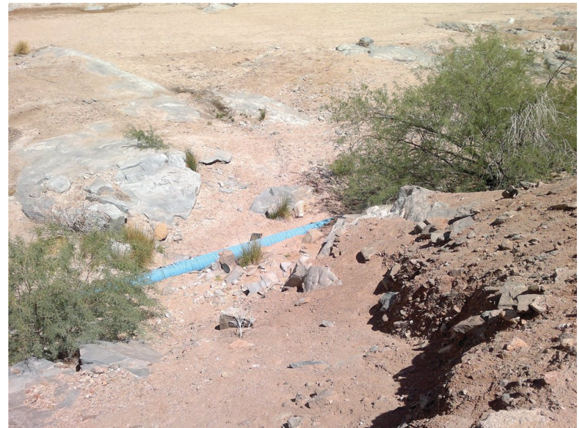
Pipeline exposed in riverbed
