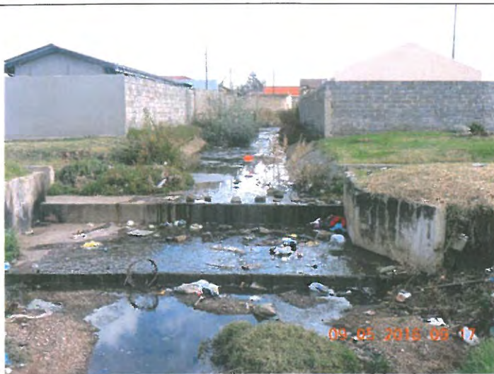
River channelized and polluted with litter. The creation of this channel has degraded vegetation and increased erosion. The channel also has sedimentation in progress.
