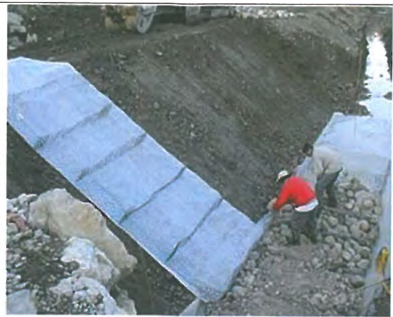
Gabion mattress can be useful at this particular slope as it is slanting
