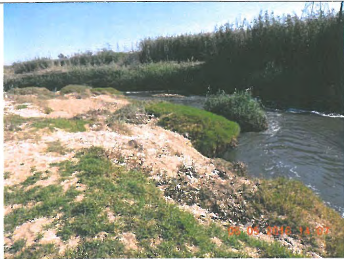
River bank erosion
