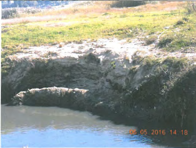
Various sections on the Klipspruit Valley Road to Chris Hani Road are eroded and need gabion support
