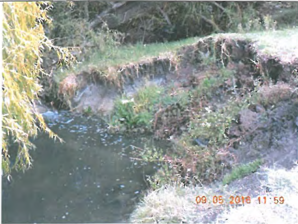
The Jabavu section highly eroded and in need of gabion support structures
