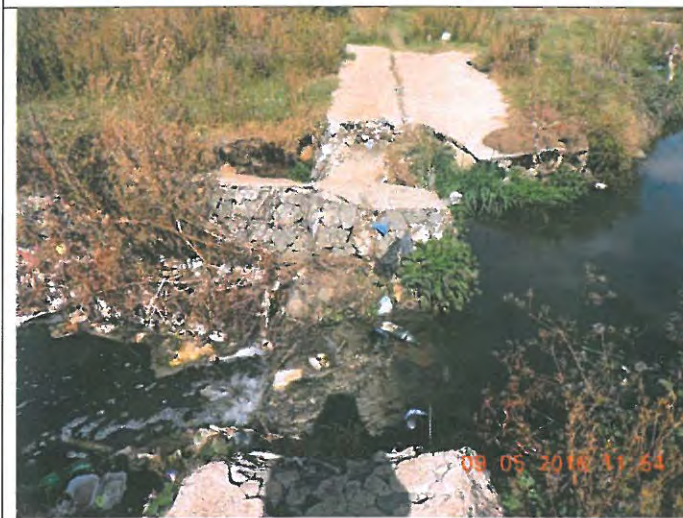
Collapsed walkway on river and vegetation
