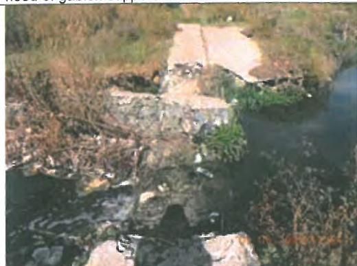
Photo E.5.1-24. Gabion collapse at the Jabavu section.
