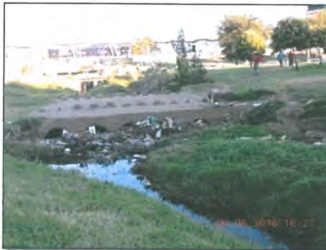
Photo E.5.1-9. Round culverts blocked with litter and silt within Thokoza Park.
