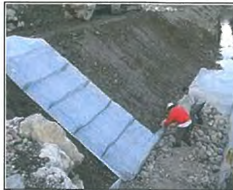
Photo 7.2-16 Gabion mattresses can be useful at this particular slope as it is slanting.
