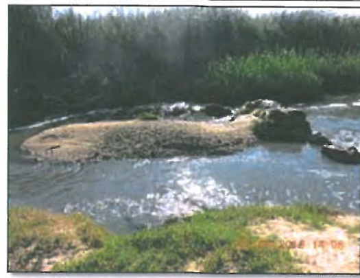
Photo 5.1-7. Sedimentation within the wetland section in Klipspruit Valley Road to Chris Hani Road section of WMU in Zone 2.
