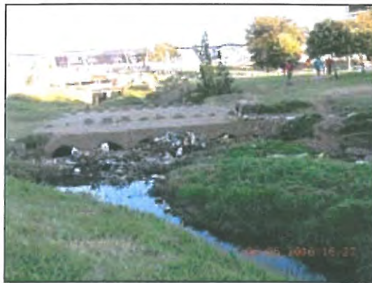
Photo 5.1-6. Round culverts blocked with litter in Thokoza Park in Zone 1.
