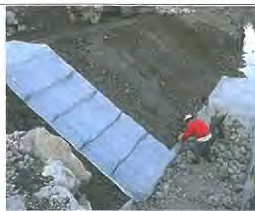
Photo E.5.1-27. Gabion mattress can be useful at this particular slope as it is slanting.
