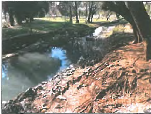
Photo 7.2-15 Gabion collapse and erosion at Dorothy Nyembe Park.
