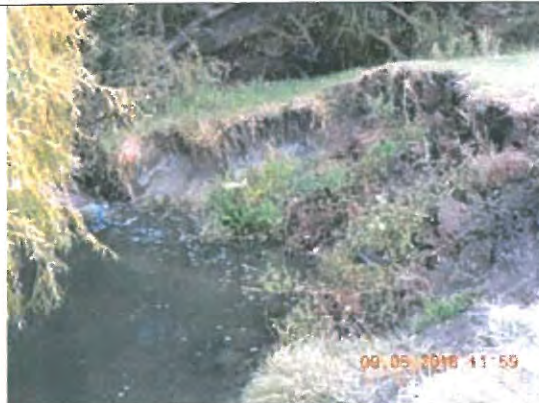
Photo E.5.1-22. The Jabavu section highly eroded and in need of gabion support structures.
