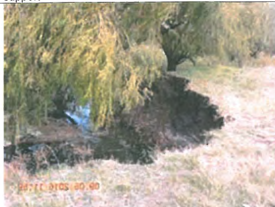
Photo E.5.1-20. The Jabavu section also has various points needing gabion structures.
