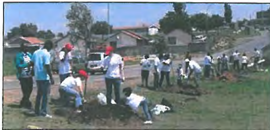
Photo E.5.1-5. An example of excavation work during tree planting and park development.
