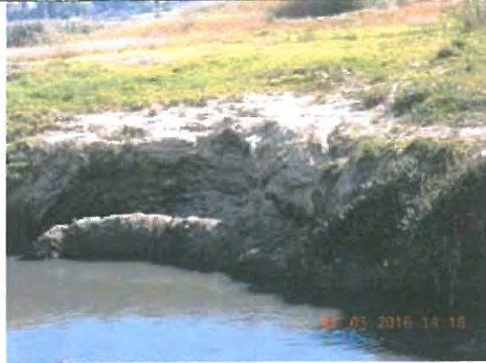
Photo E.5.1-18. Various sections on the Klipspruit Valley Road to Chris Hani Road are eroded and need gabion support
