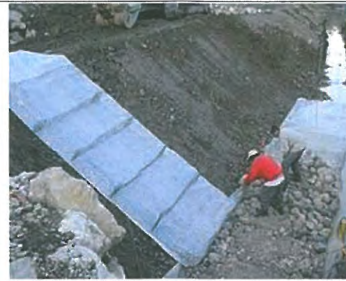
Photo E.5.1-23. Gabion mattress can be useful at this particular slope as it is slanting.
