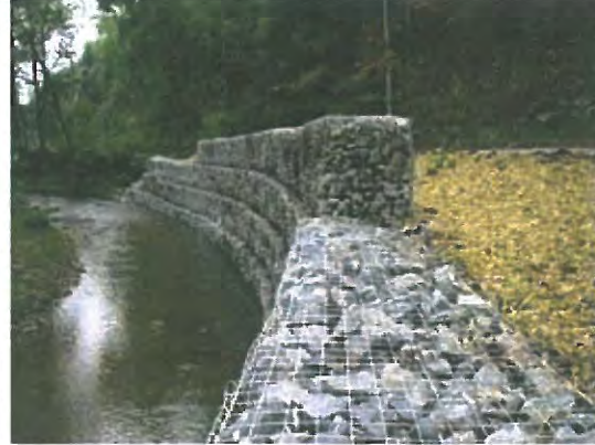
Photo E.5.1-19. Gabion baskets can be used to stabilise banks
