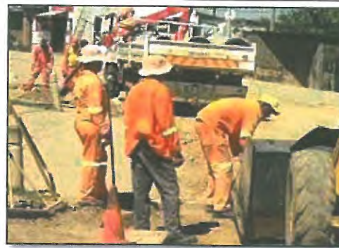
Photo E.5.1-4. Example of installation of excavation for installation of cement fence structures.
