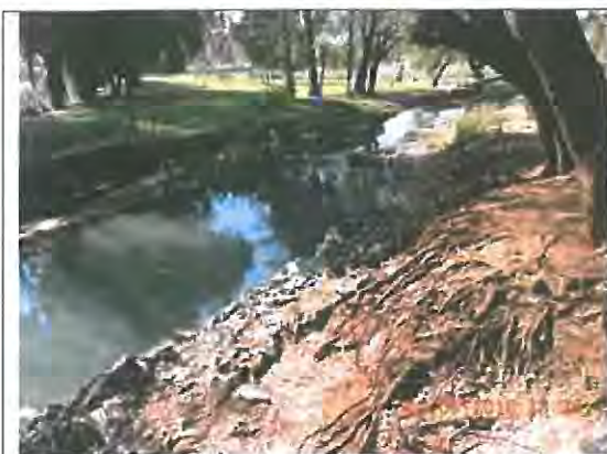
Photo E.5.1-26. Gabion collapse and erosion at Dorothy Nyembe Park.
