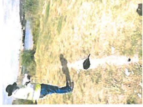
Photo B. 2-3. (WP 917): Damaged Storm water outlet infrastructure.
