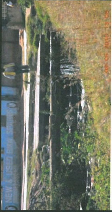
Leaking sewage pipe above tributary feeding into Dorothy Nyembe Park.
