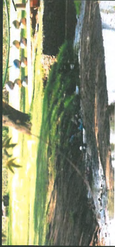
Erosion and sedimentation at Dorothy Nyembe Park entrance.
