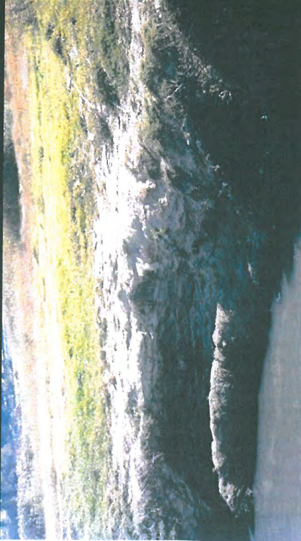
Various sections on the Klipspruit Valley Road to Chris Hani Road are eroded and need gabion support - Zone 2
