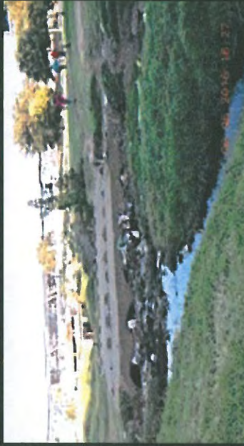
Round culverts blocked with litter in Thokoza Park in Zone 1.
