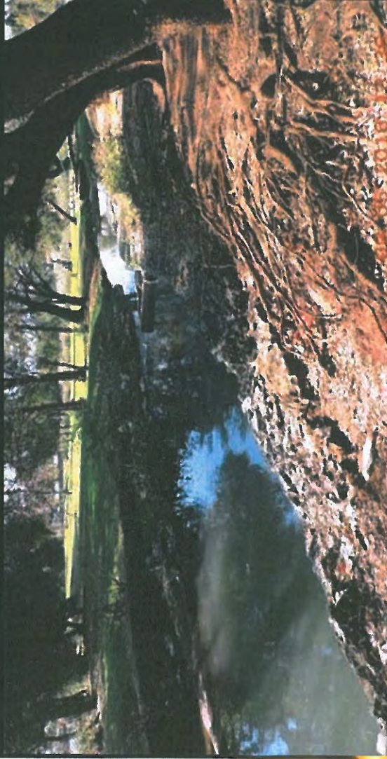
Gabion collapse and erosion at Dorothy Nyembe Park – Zone 3
