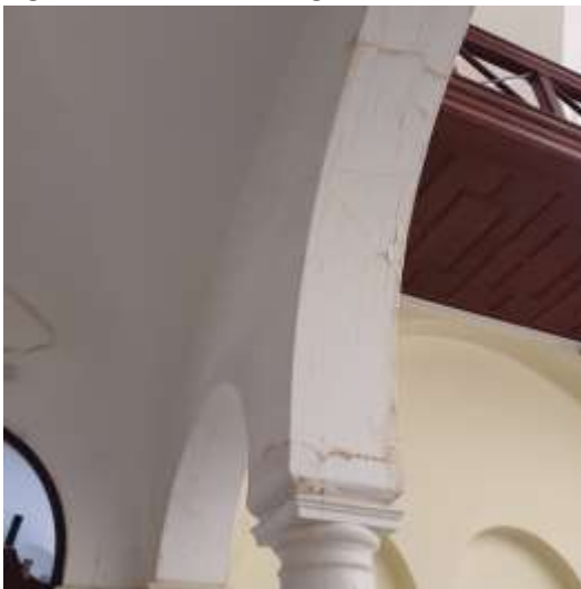
Fig 13 : Ground floor - Damages to ceiling and arches
