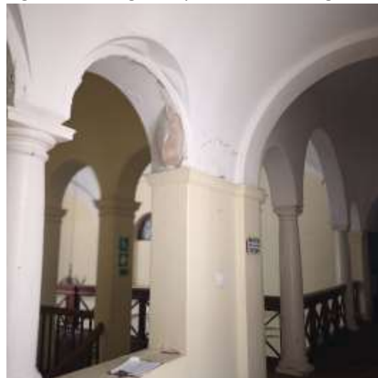
Fig 14 : First floor – Damages to the arches
