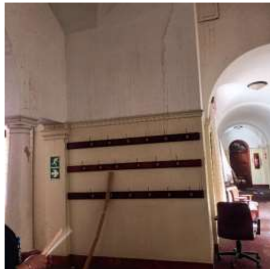
Fig 16 : First floor – Damages to the walls
