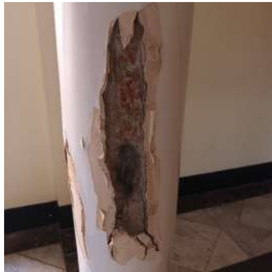
Fig 4 : Close-up of damaged column
