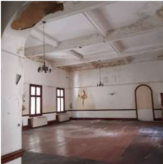
Fig 20 : First floor – Damages in Art Gallery
