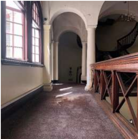
Fig 19 : First floor timber walkway – water damaged carpet – timber flooring below
