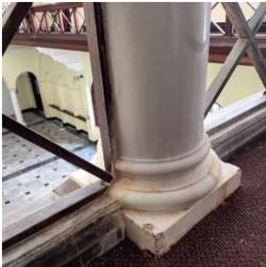
Fig 9 : First floor - Damaged base of column
