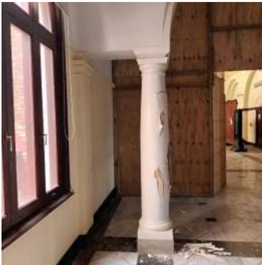
Fig 3 : Ground floor – damaged column
