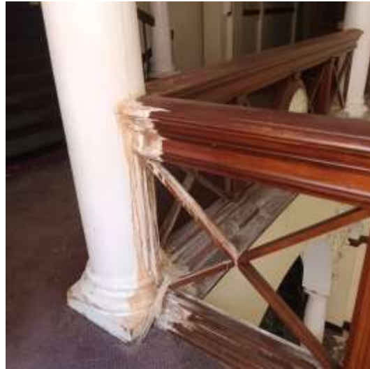
Fig 18 : First floor – Damages to handrail
