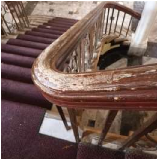
Fig 17 : Stairs – damages to handrail
