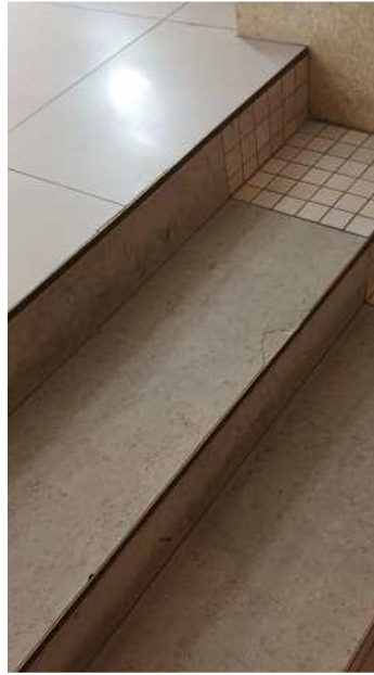
Figure 7 Broken Floor Tiles
