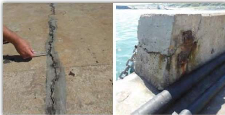
Figure 9: Structural cracks to be repaired
