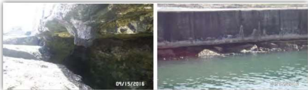
Figure 3: Voids to be filled and undermining to be capped
