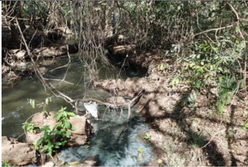
Bank collapse and under-cutting
