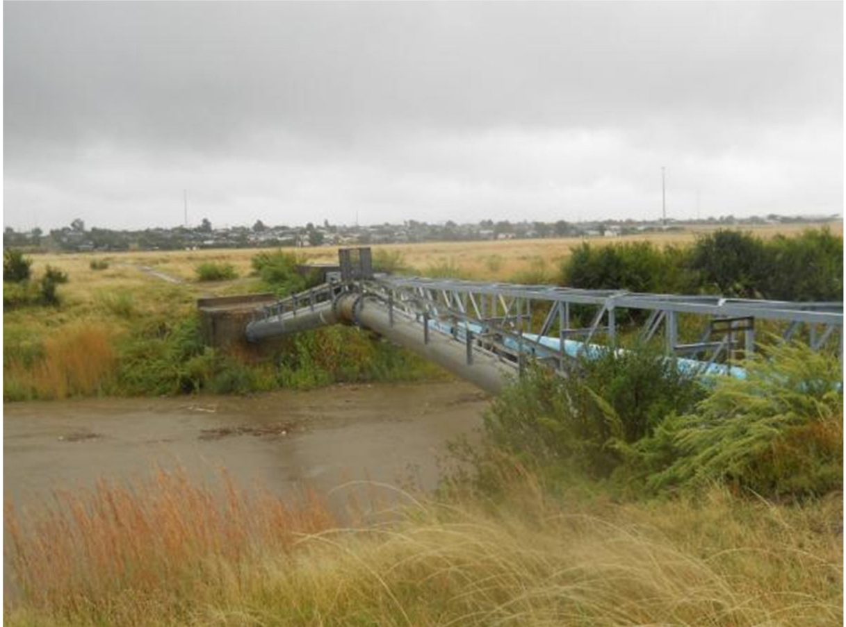
Figure 6.5 Existing pipeline crossing the Klein Modder River. No outcrops, no fossils observed (GPS: S29° 15' 10,4" E26° 41' 59,5")
