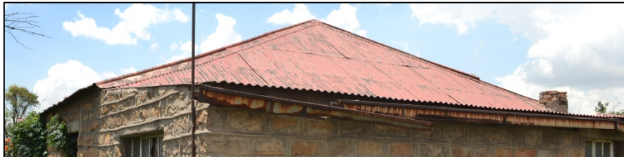
Figure 41. Some effort was made to mount gutters but without downpipes. Water was directed to a single detached corrugated iron water reservoir (Photograph: M. Naude 2016).
