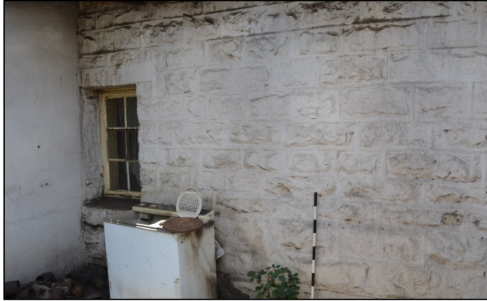
Figure 7. White washed sandstone wall at the back of the dwelling where a veranda was later added (Photograph: M. Naude 2016).
