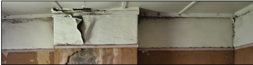
Figure 25. Gypsum boarding with pine planking and sealed with molded cornices (Photograph: M. Naude 2016).
