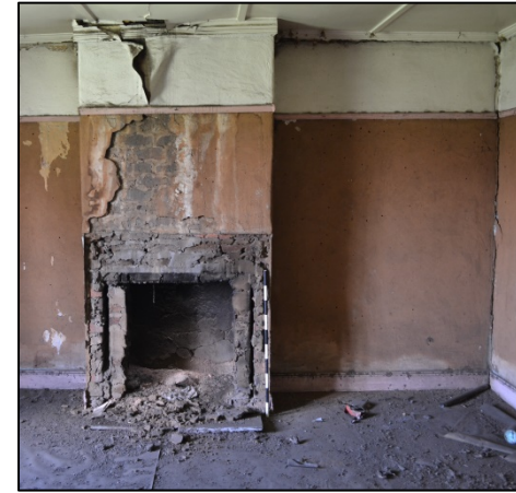
Figure 20. Protruding fire place in the lounge. the mantelpiece has been removed (Photograph: M. Naude 2016).
