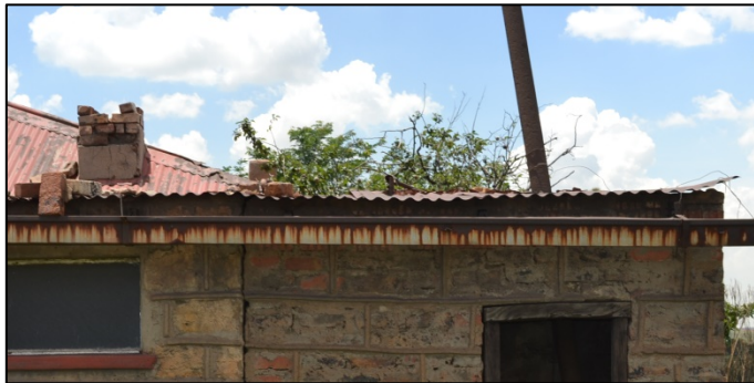
Figure 18. Sheet iron chimney pipe leading from the boiler room (Photograph: M. Naude 2016).
