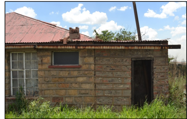
Figure 15. The most recent addition was this boiler room. The small extension was also constructed with stone but applied in a different style. The new room was clearly demarcated but the pointing was applied to blend with the pointing of an earlier addition (Photograph: M. Naude 2016).
