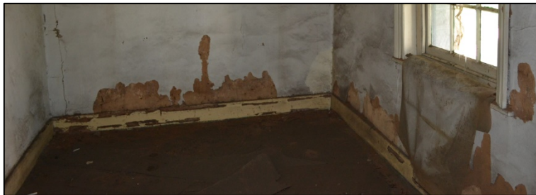
Figure 10. Rising damp in the room adjacent to the front veranda (Photograph: M. Naude 2016).
