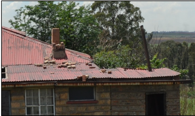
Figure 17. General position of the three chimneys and chimney pipes (Photograph: M. Naude 2016).
