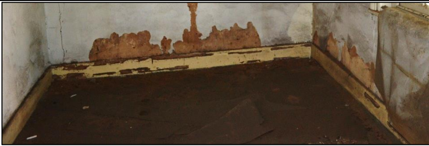
Figure 2. Floor of the front room facing the front stoep - note the rising damp problem just above the skirtings (Photograph: M. Naude 2016).
