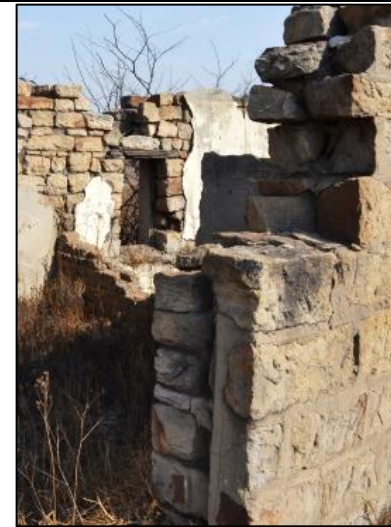
Figure 17. Remains of a door where the frame has been removed.
