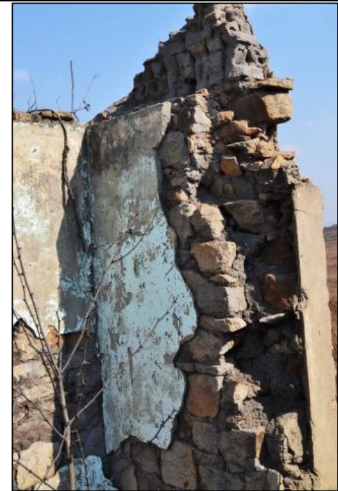
Figure 13. Sundried clay bricks on top of the sandstone wall, define the triangle of the remains of the gable
