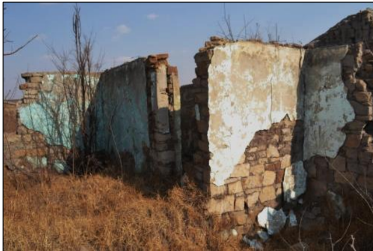
Figure 10. Painted cement and sand plastering along the interior of the original exterior walls
