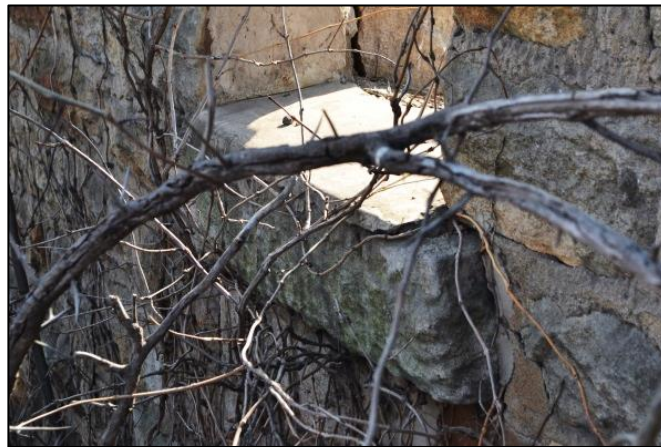
Figure 8. Projecting dressed sandstone window sill neatly incorporated as part of the exterior walling
