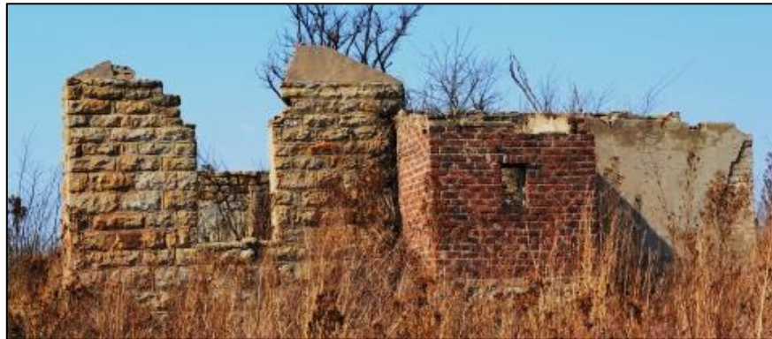
Figure 3. South-eastern facade with gable and recent toilet and bathroom additions done in red bricks.
