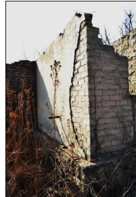
Figure 12. Sundried bricks exposed after the plastering have been washed off the addition along the southwestern facade
