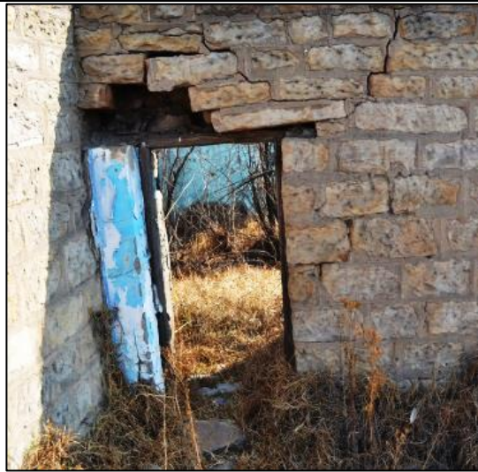
Figure 16. Remains of a single door frame
