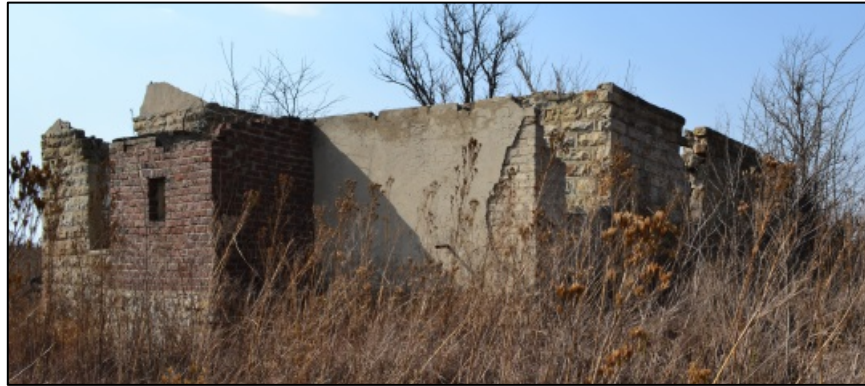
Figure 4. This used to be the principal facade with gable and stoep where the red brick and plastered room were added to form the bath room and toilet
