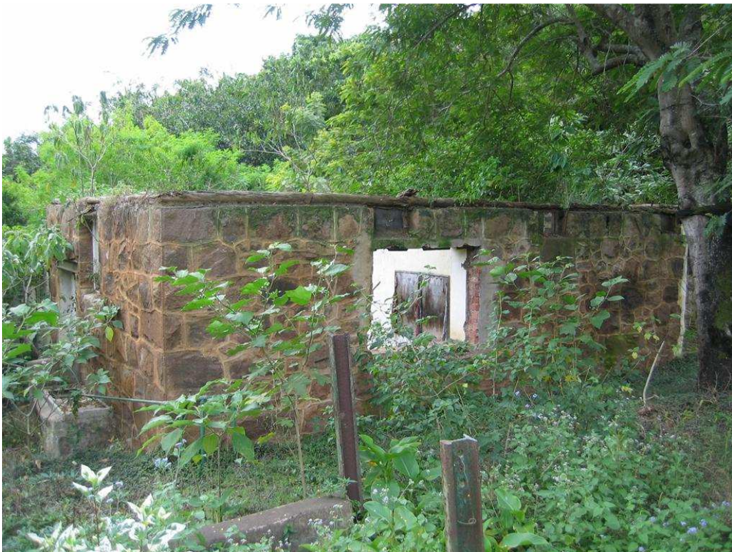
Plate Error! No text of specified style in document.-1: Derelict stables requiring demolition application
