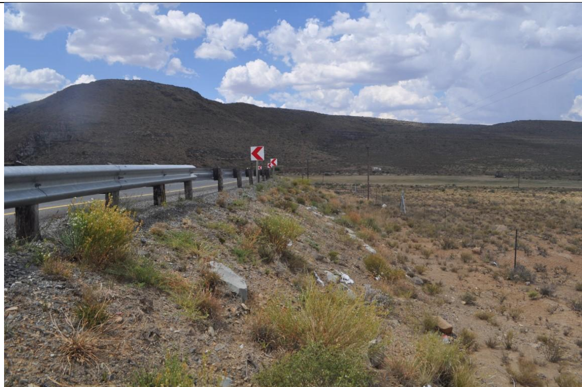
Road has been lifted / Guardrails / No Access to "road" shown on Google Earth Height difference from top of embankment to bottom +/- 3m
