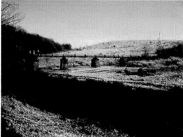
Sewage pipe in rural area
