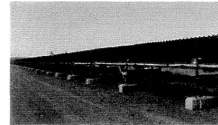
Example of typical coal conveyor from the side
