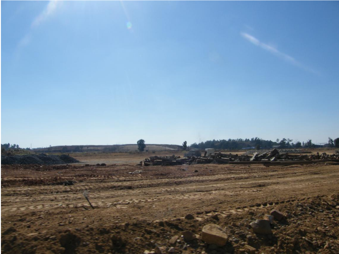
Photograph 15: Material stockpiles for the railway upgrade by Transnet – at the southern part of the site
