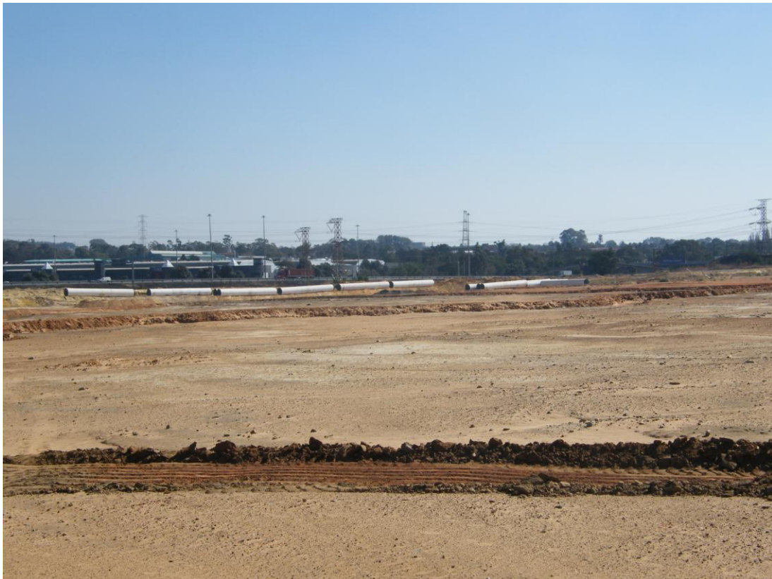
Photograph 8: Looking west from the middle of the site - Randwater pipeline construction at the western boarder of the site
