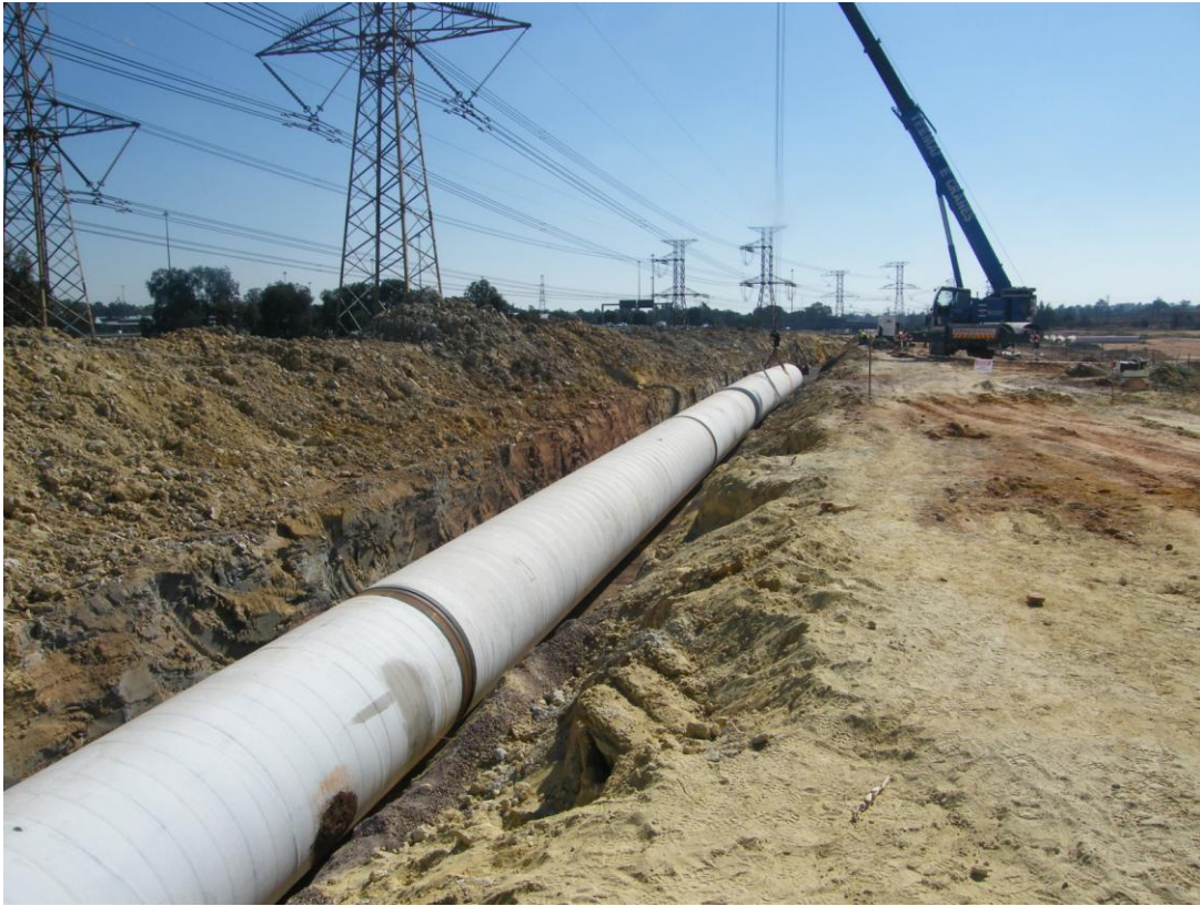
Photograph 9: A trench for the Rand water pipeline at the western border of the site
