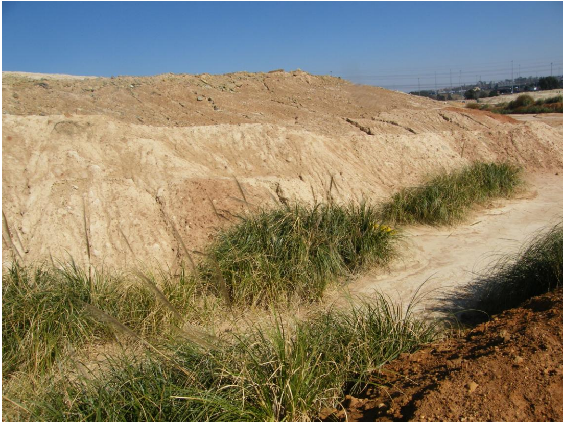
Photograph 3: Stormwater channel - from the south to the middle part of the site
