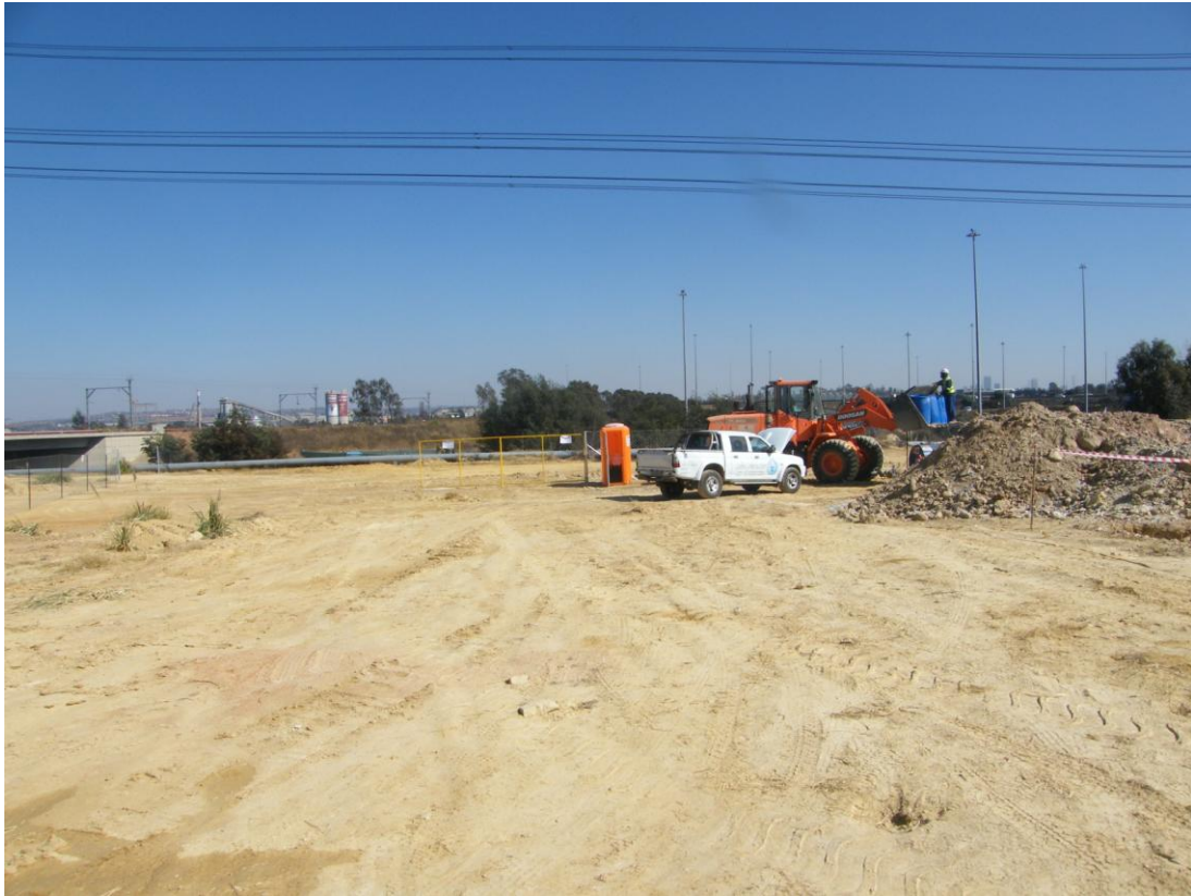
Photograph 7: Looking west from the middle of the site - Randwater Pipeline construction site
