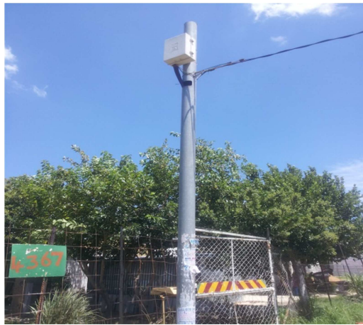
Existing Powerlines, lighting control box and transformer adjacent to the proposed road
