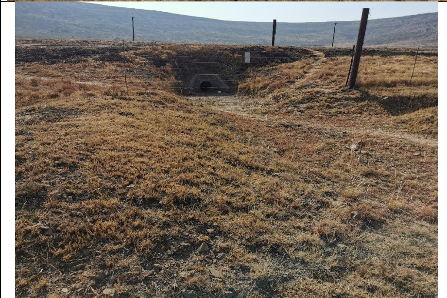
Photo of culvert running underneath the N3 national road adjacent to the site.
