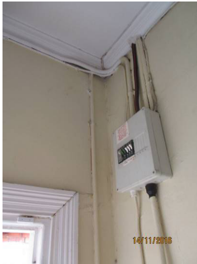
Main Distribution Board
