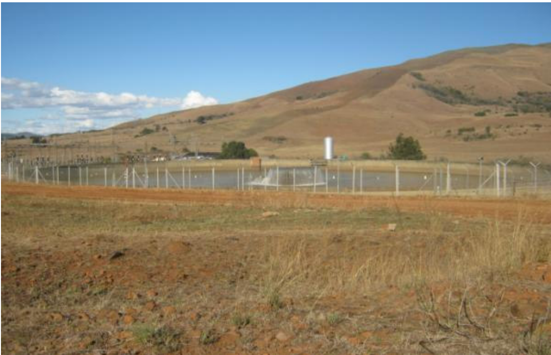
Figure 6 Northerly direction of Bosloop substation
