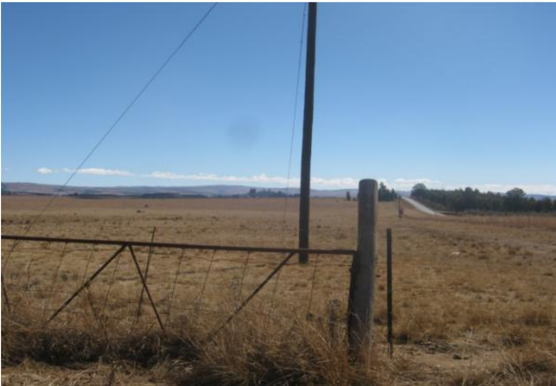
Figure 12 Westerly direction of the powerline route
