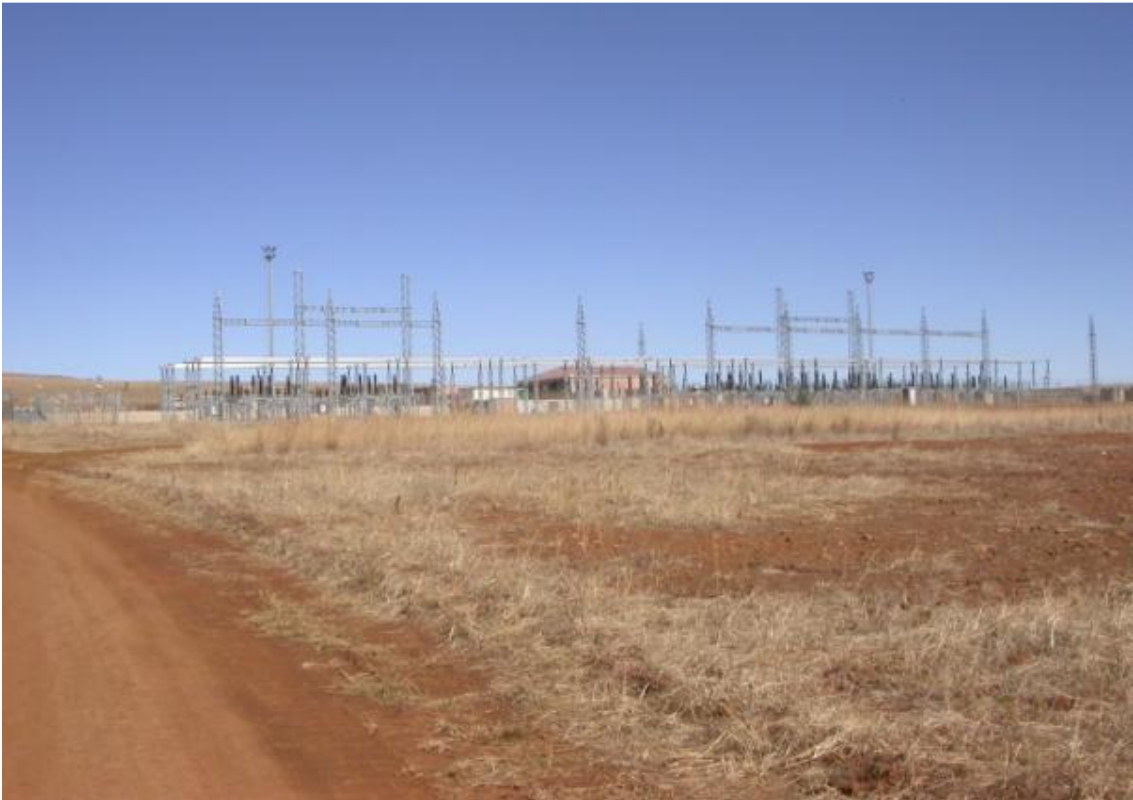
Figure2 Gumeni Substation in the westerly direction
