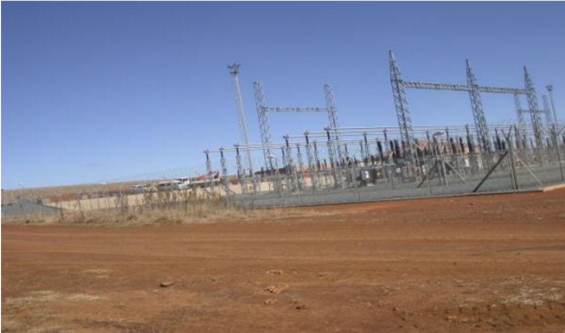
Figure 1 Gumeni Substation in the southerly direction
