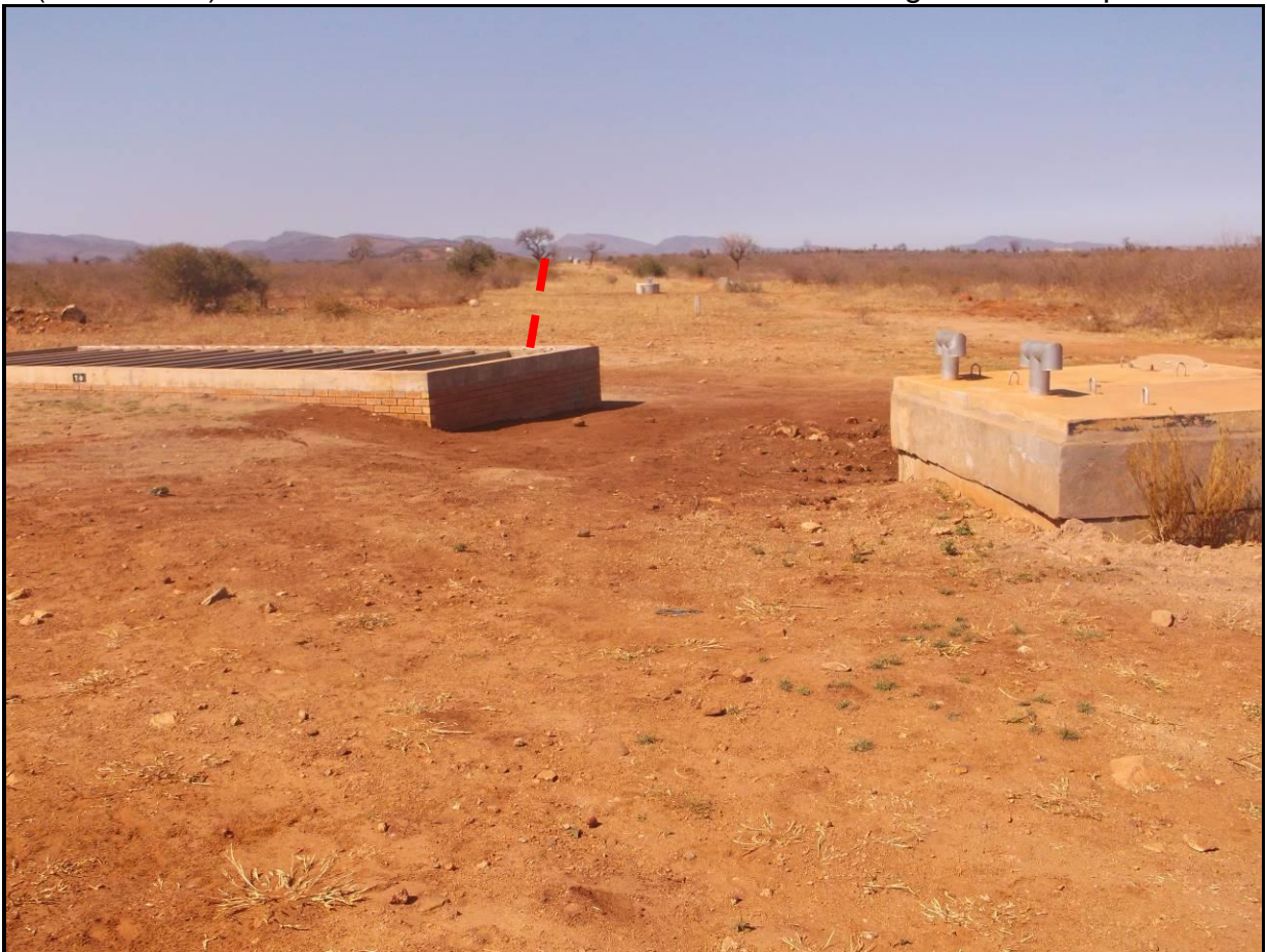
Figure 10: View of end of the pipeline route at the connection point with the existing pipelines near Tshamahansi Village
