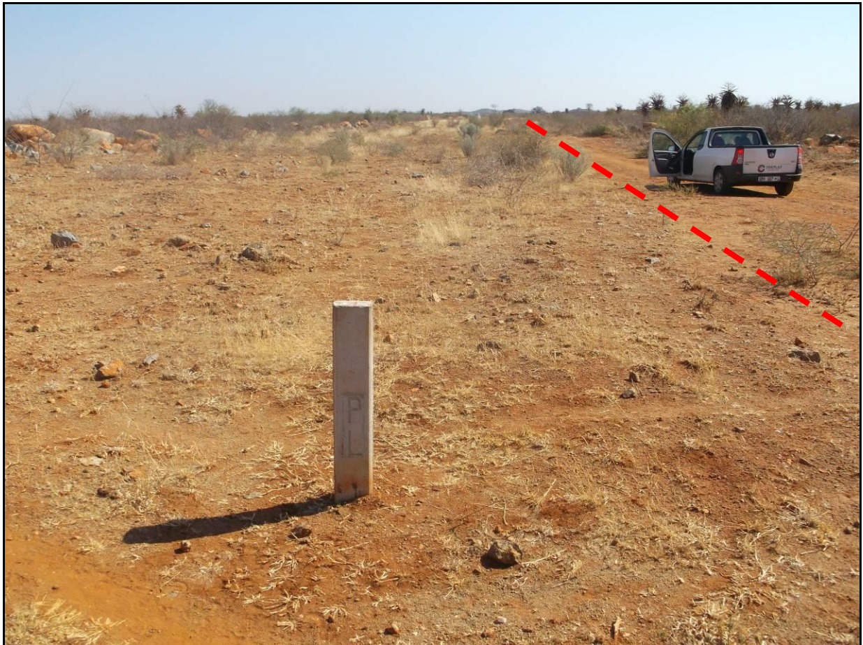
Figure 8: View of proposed pipeline route next to existing pipeline and access road
