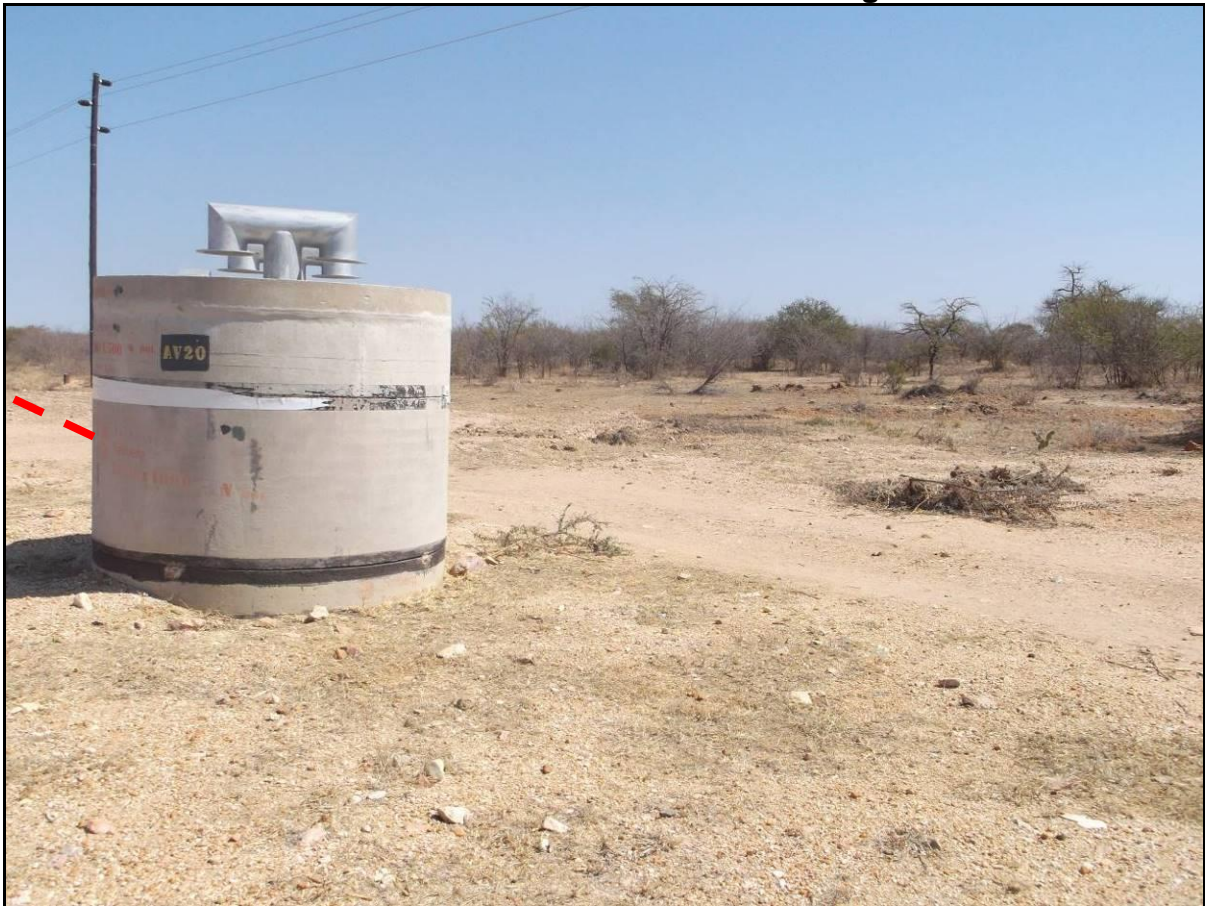
Figure 11: View of start of pipeline route at the connection point with the existing pipeline near Witrivier/Phafola
