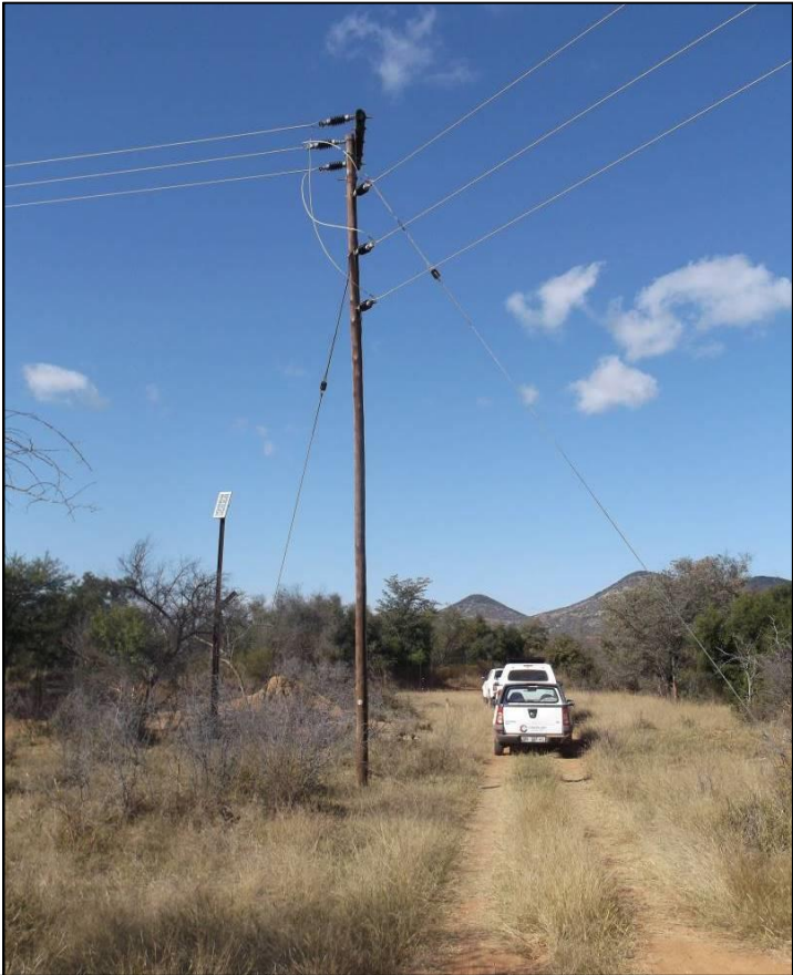
View of electricity connection point adjacent to the site.
