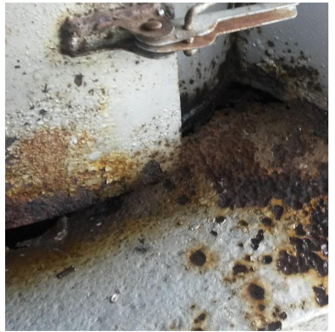
Photo 4: Rust on the chimney
