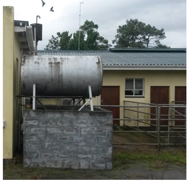
Photo 2: Diesel storage tanks outside clinic
