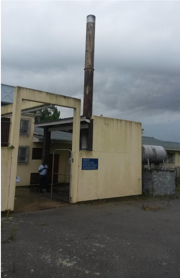
Photo 5: View of the incinerator's chimney indicating the rust
