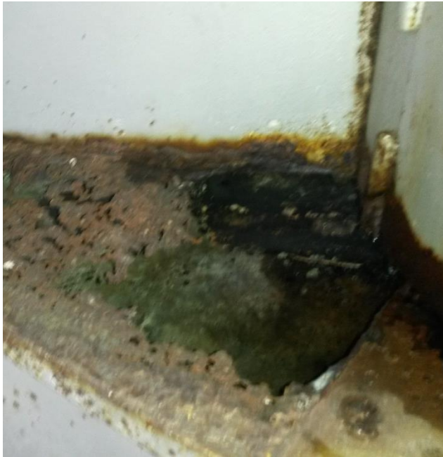
Photo 3: Rust at the base of the chimney
