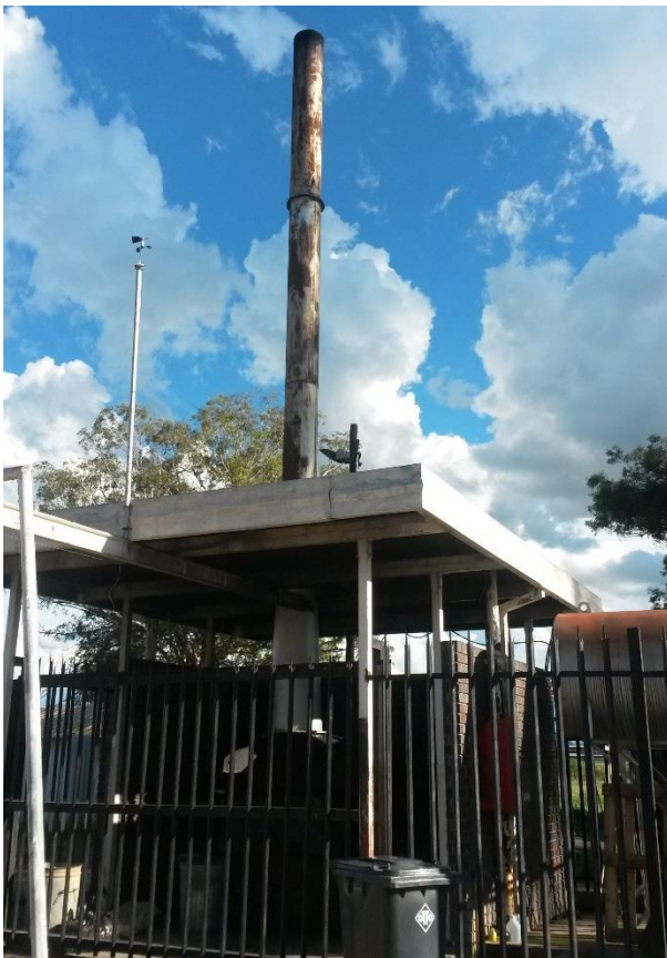
Photo 3: View of the incinerator's chimney indicating the rust
