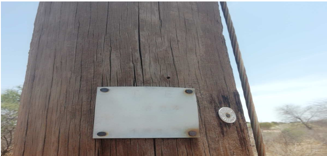
Figure 2: Pole number where the power will be connected from
