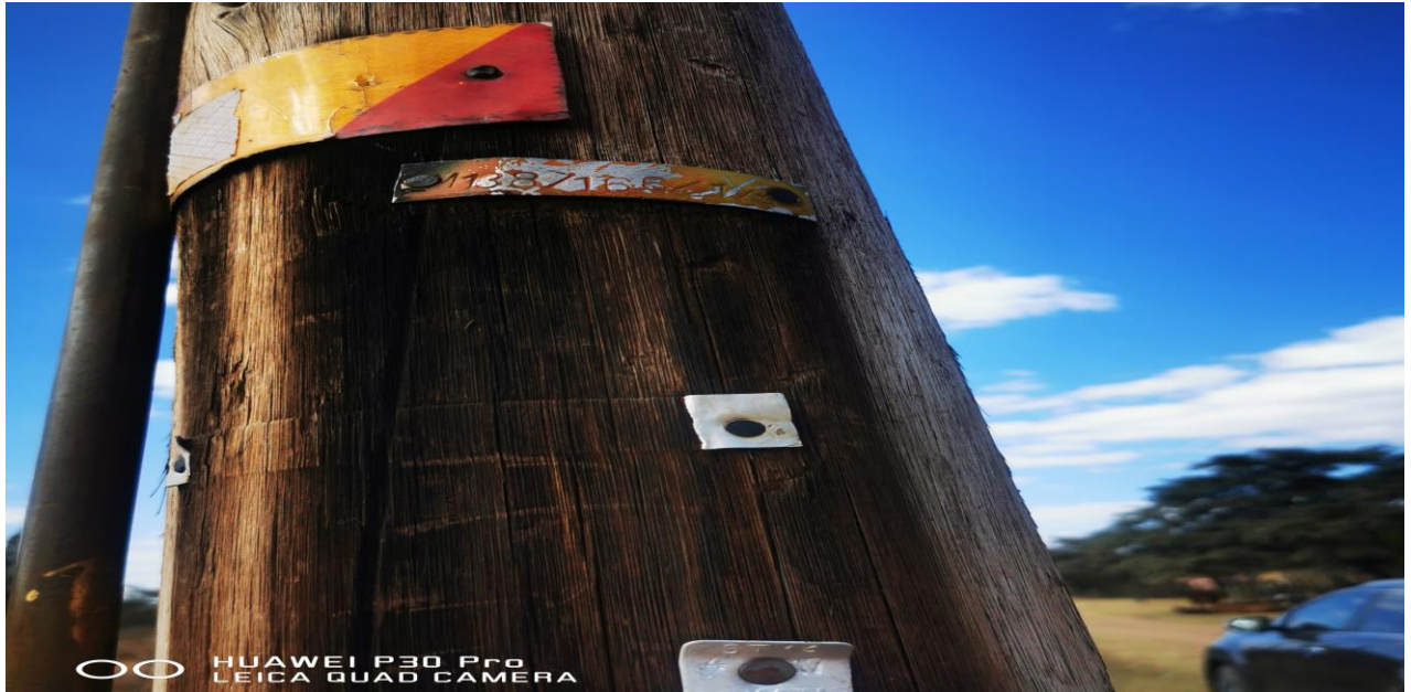
Figure 1: Existing pole number where the electricity will be supplied from
