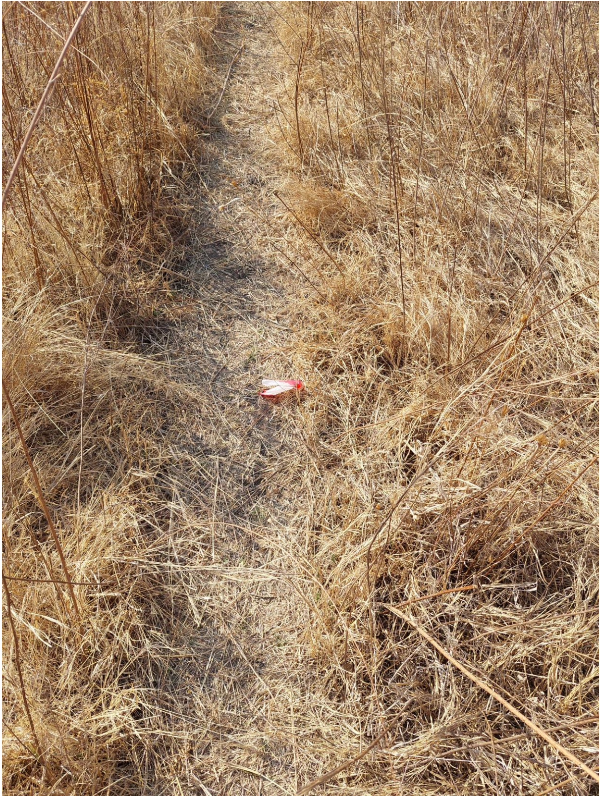
PICTURE SHOWING ANOTHER PROPOSED POLE POSITION
