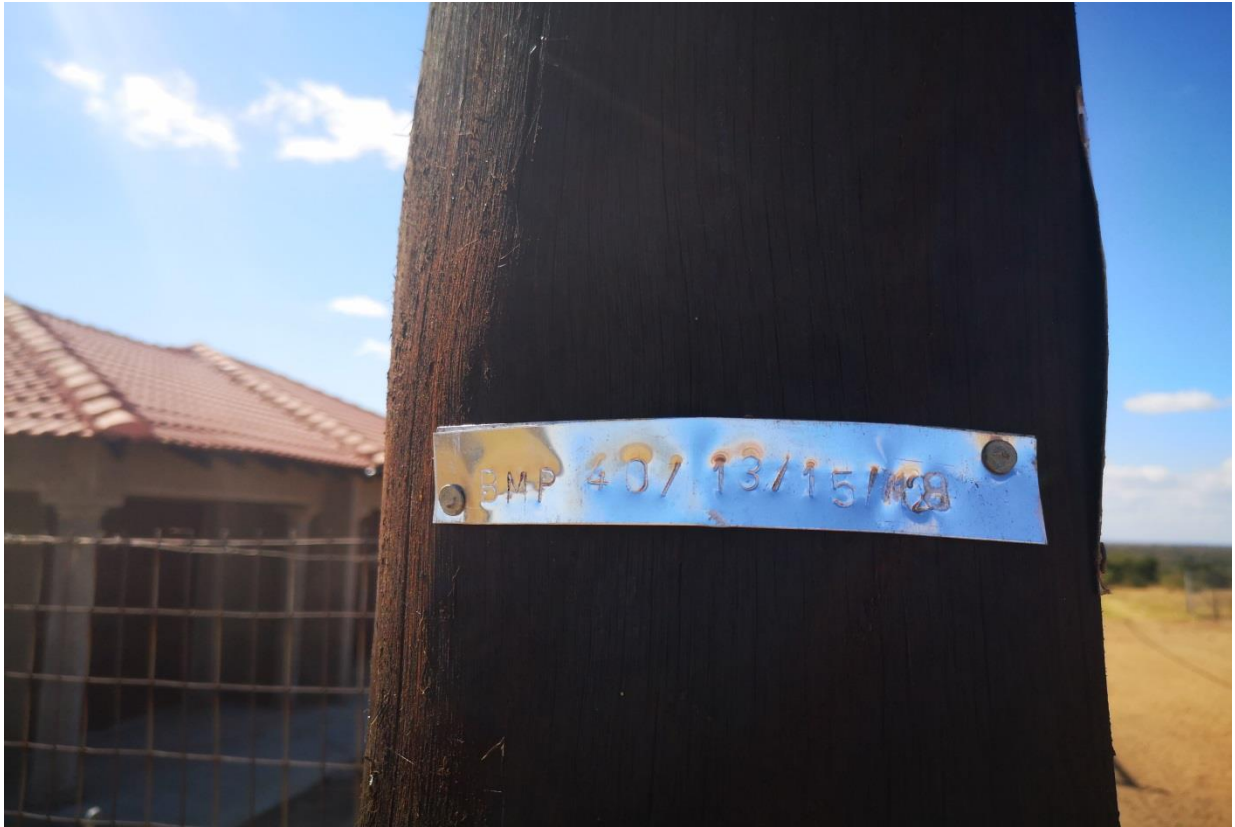
Picture 1: Shows the existing pole number on site
