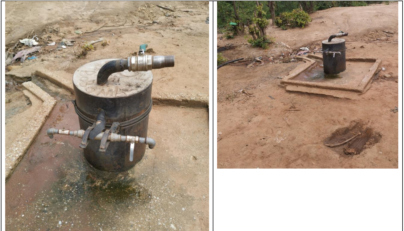
Figure 7 Unauthorised water bulkline connection structure
