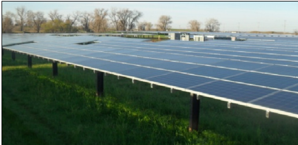
Figure 6: Frontal views of the PV arrays mounted on horizontal 1-axis tracker
