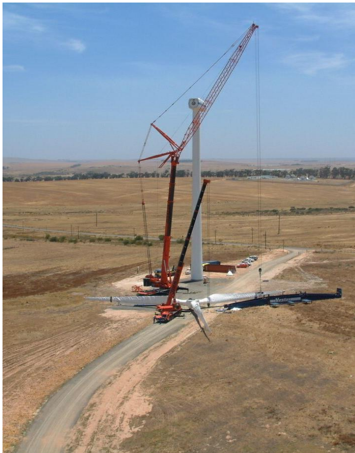
Figure 3.6: Photograph illustrating the laydown areas required during the erection of a turbine (photo courtesy of Eskom)
