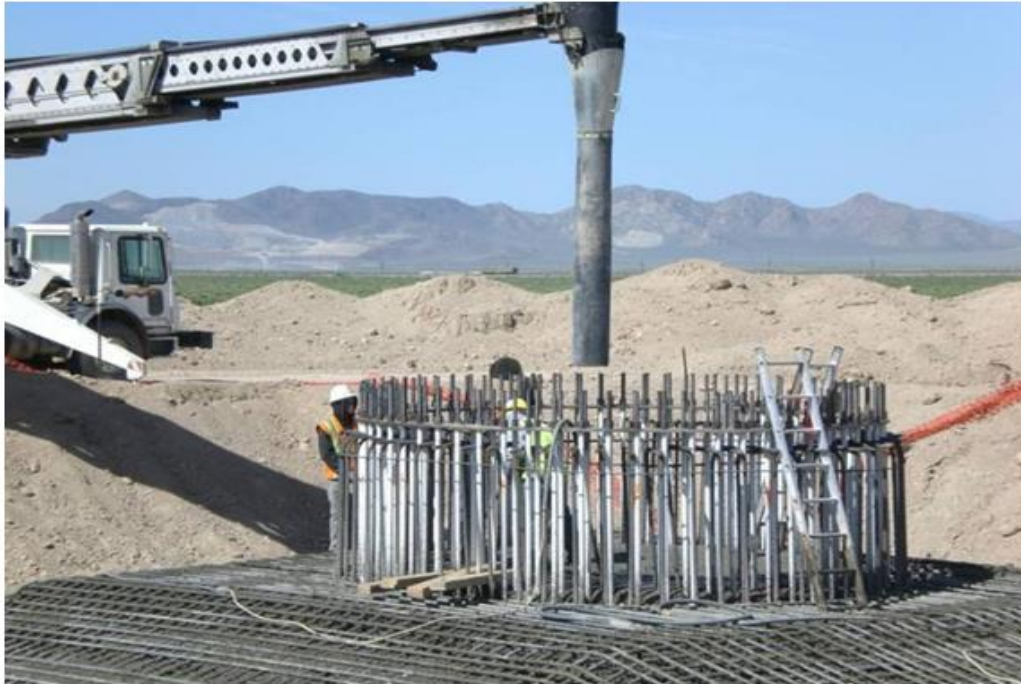
Figure 3.2: Photograph illustrating the construction of the foundation for a wind turbine (photo sourced from www.blm.gov )
