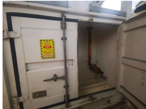
Plate 2: Opening of aboveground self-bunded paraffin storage tank
