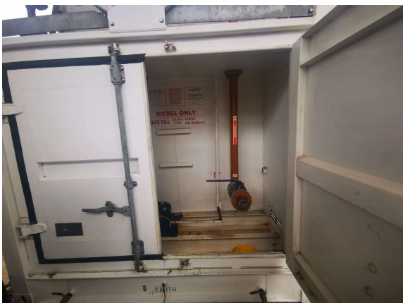
Plate 4: Opening of aboveground self-bunded diesel storage tank
