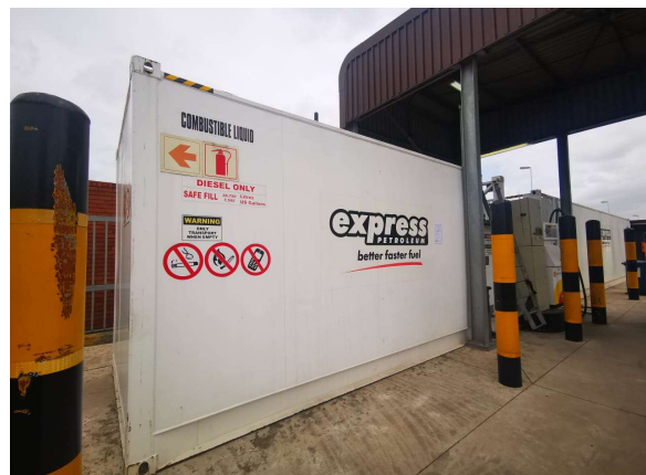
Plate 3: 28 750 litre diesel storage tank
