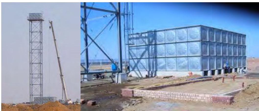
Figure 4.8.9.6.1(a): Potable Water Storage at Shaft Complex
