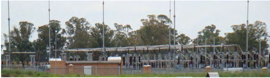
Figure 4.8.1.5(a): Electrical Sub-Station at iThemba Lethu Shaft
