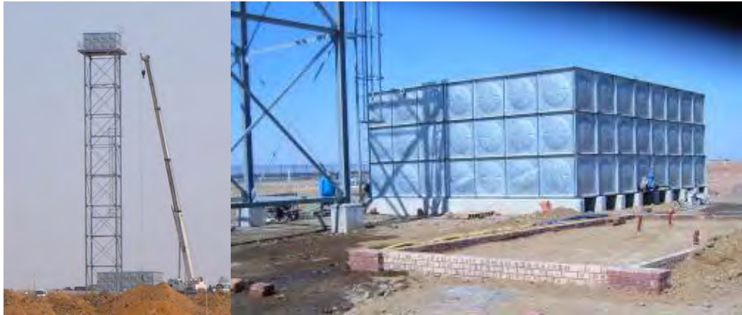
Figure 4.8.7.1(a): Potable Water Storage at Shaft Complex
