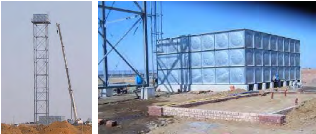
Figure 5.14.2.1(e): Potable Water Storage at Shaft Complex
