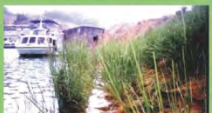
China - partially submerged vetiver grass used to stabilize the draw-down slope of a reservoir in Guangdong Province
