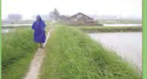
Vietnam - cyclone damage to sea dykes is a major problem. VS has been applied successfully for disaster mitigation
