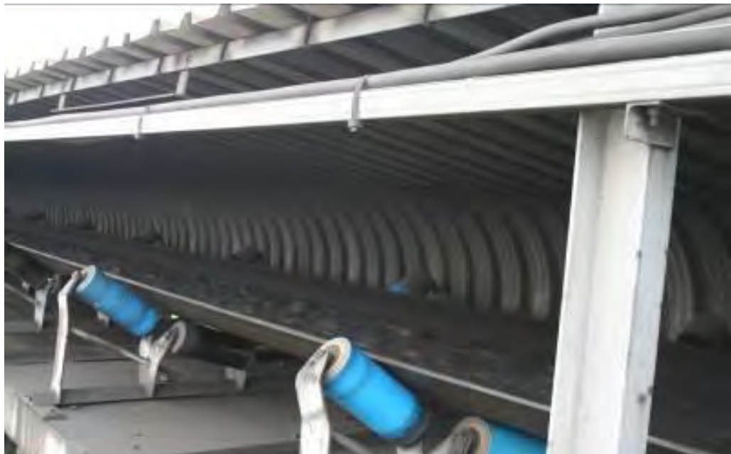
Figure 2.4(a): Conveyors will use plastic idlers and will be covered to prevent rain wash, as well as dust and noise propagation
