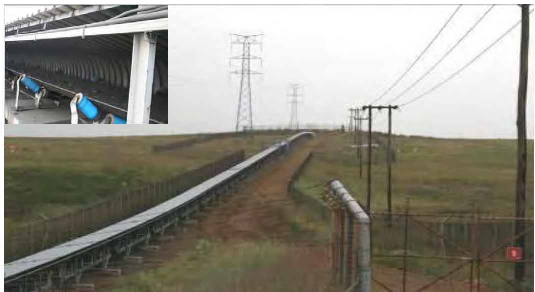
Figure 5.1(d): A Typical Overland Coal Conveyor
