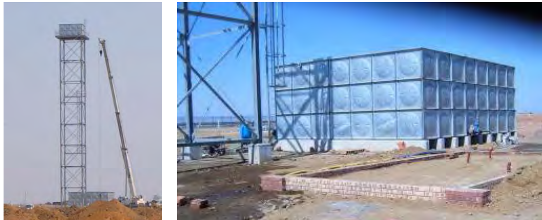
Figure 5.1(e): Potable Water Storage at Shaft Complex
