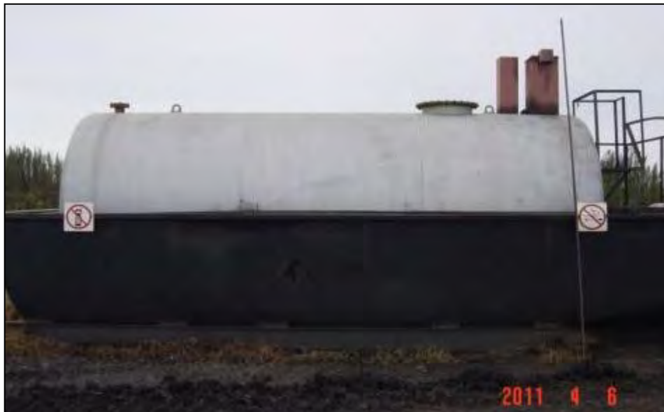
Figure 3.1.5.2.7 (a): Typical Diesel Storage Tank – note the Spillage Bowl.
