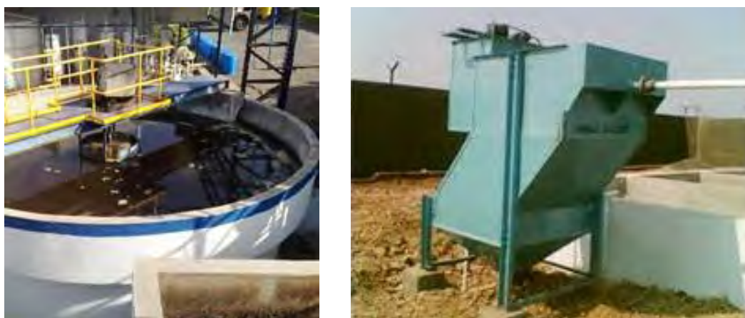
Figure 3.1.5.17.4 (e): Conventional Circular and Lamella Softening Clarifier
