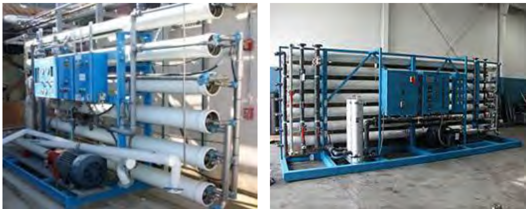
Figure 3.1.5.17.4 (d): Reverse Osmosis Treatment Skids
