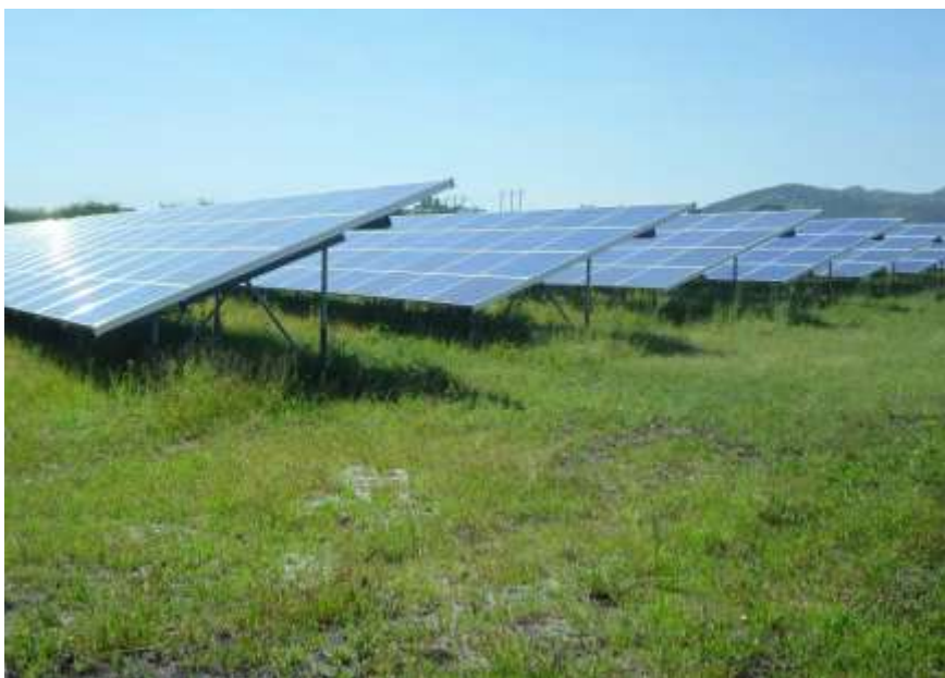
Figure 2.4: Photo showing view of photovoltaic panels
