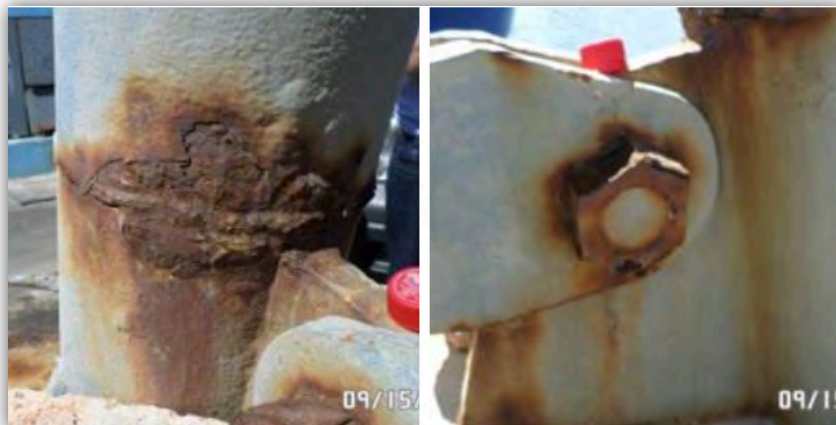
Figure 1.2.3.1d: Damage to vertical members and fixing detail
