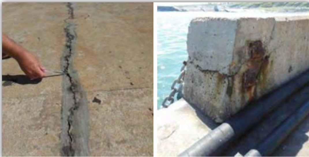
Figure 1.2.3.1b: Structural cracks to be repaired
