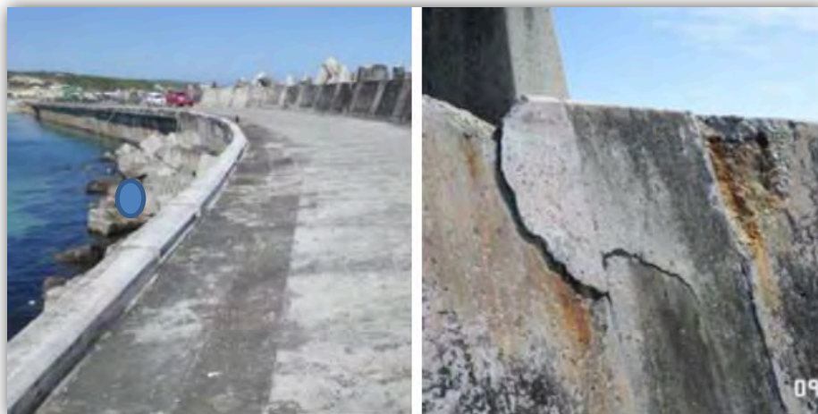
Figure 1.2.2.2: Damage to Breakwater 3 and area where water is allowed through (see blue circle)
