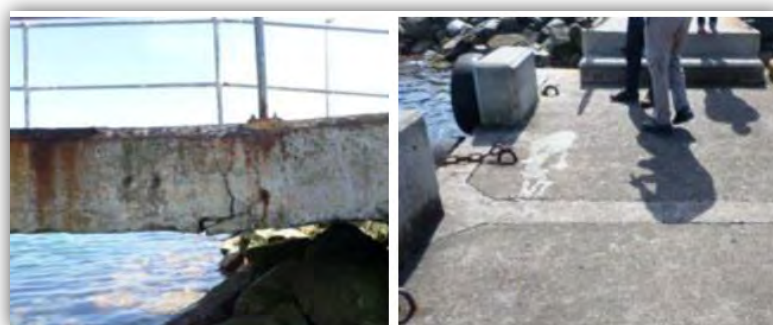
Figure 1.2.2.4: Damage to Jetty 2
